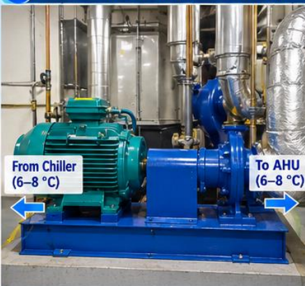
3 Chilled Water Pump (Actual Unit)
