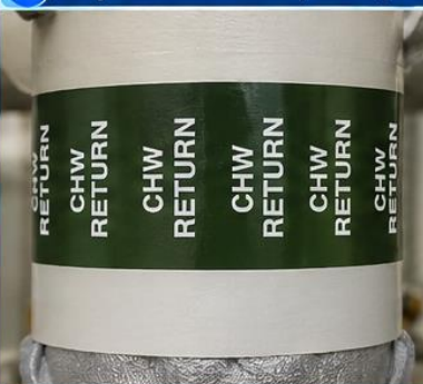
5 Pipe Identification (Return)
