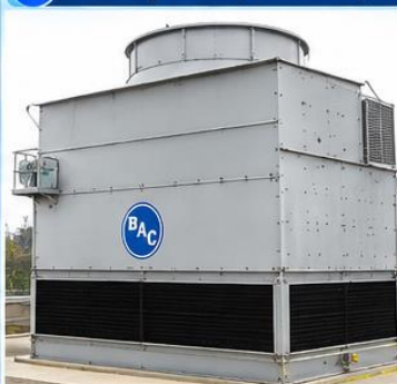
8 Cooling Tower (Actual Unit)
