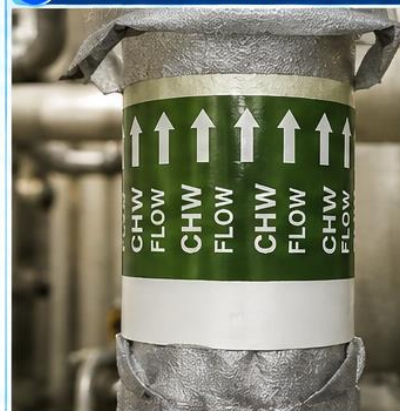
4 Pipe Identification (Chilled Water)
